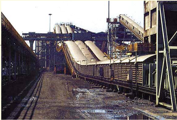
Troughed belt conveyer
