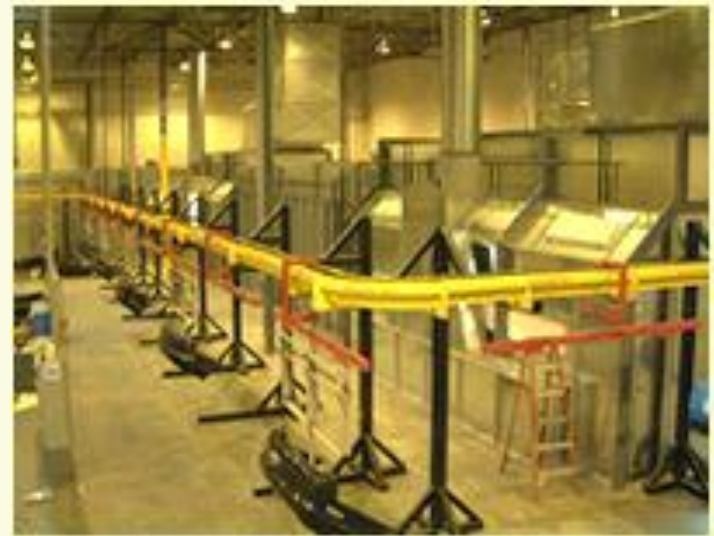
Tow line conveyer
